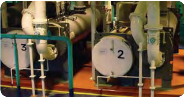
CEMS Engineering built a control system to reduce energy use of industrial air chillers by 30 percent.
